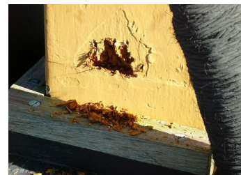
Wooden parts are susceptible to rotting
